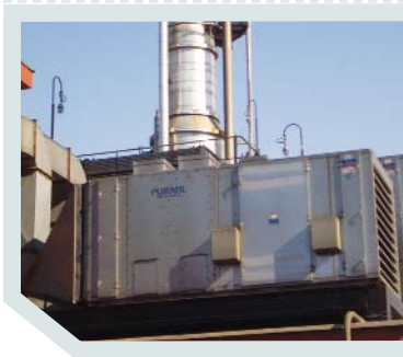
PURAFIL DEEP BED SCRUBBER AT TUPRAS IZMIT REFINERY IN TURKEY
